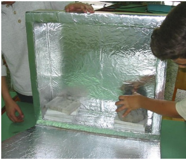
Photo 7: We have constructed the reflector and now we stick it on one of the sides of the cooker base ...
