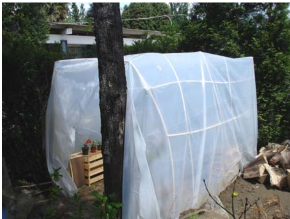
Photos 25, 26 & 27: Pupils building their greenhouse out of plastic tubes affixed to bases of concrete and with plastic film all around ( Escola Antré Soares, PT ).
